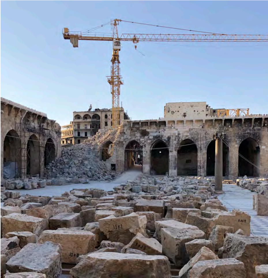
Figure 10.6 Damage to the Great Umayyad Mosque of Aleppo, including damage to the minaret. Image: Francesco Bandarin
