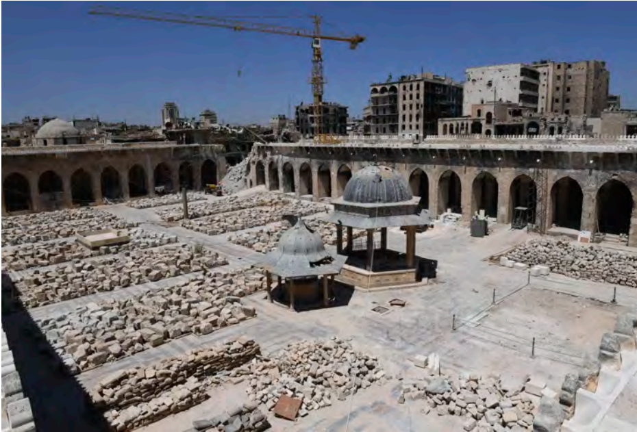
Figure 12.2 Restoration work underway at the Great Umayyad Mosque in the Old City of Aleppo, 14 August 2018. A crane stands over the rubble of the toppled eleventh-century minaret, whose stones have been catalogued and organized in the mosque's courtyard. Image: George Ourfalian / AFP / Getty Images
